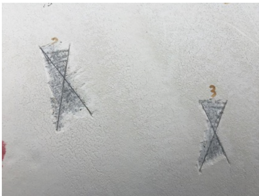
Figure 4 – Cross-cut adhesion of EonCoat – June 2018 after 4 months of being insulated and in service.
